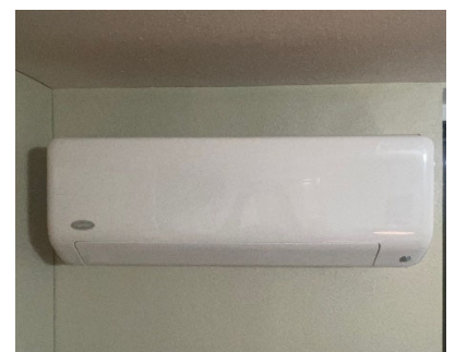
New AC/Heat Pump Unit
